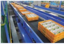
Material handling system delivery and installation project for food distribution center (South Korea)
