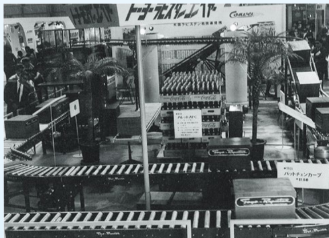
Rapistan conveyor (delivered to the Harumi Post Office of the Ministry of Posts and Telecommunications)
