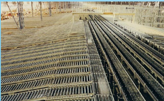
Rapistan conveyor system delivered to the Fuchu Distribution Center of Seiyu Store
