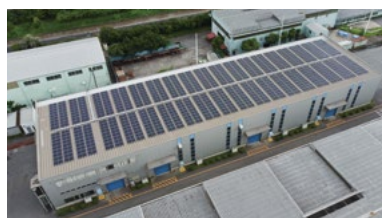
Solar power generation equipment at the Chiba Office
